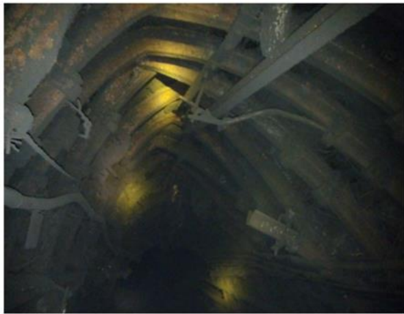
Figure 1. Deformation and subsidence in transport tunnel at the Mong Duong mine.
